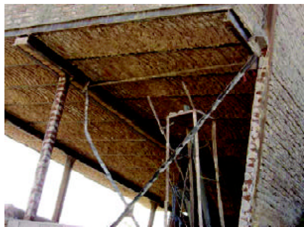
Figure 13. Buckling of bracing and connection damage.
