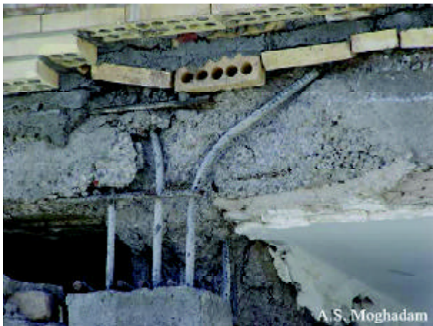
Figure 14. Poor detailing in connection.
