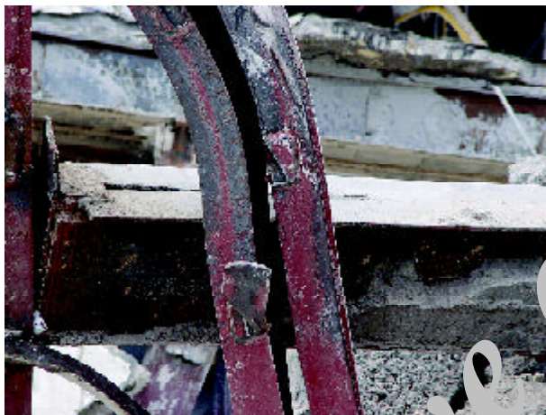
Figure 14. Rupture of battens in a shopping center.
