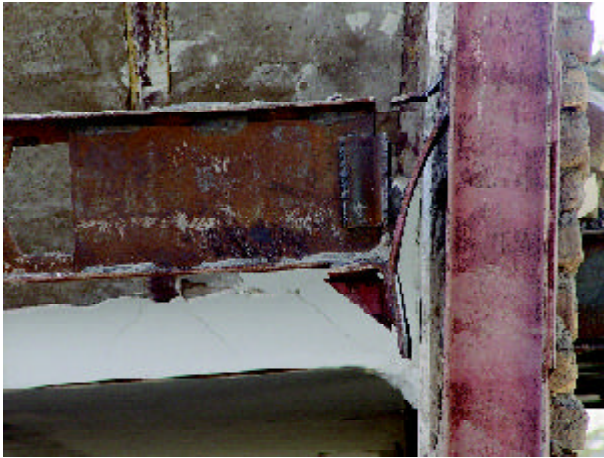
Figure 5. Weld rupture of web and top angle of connection and separation of column plate.
