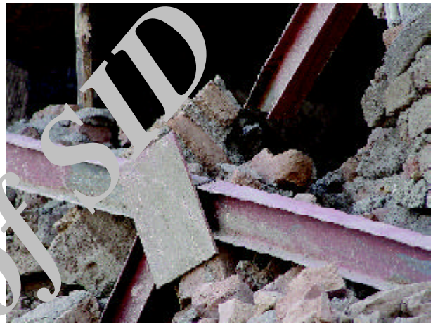
Figure 3. Rupture of connections in concentrically X bracing.
