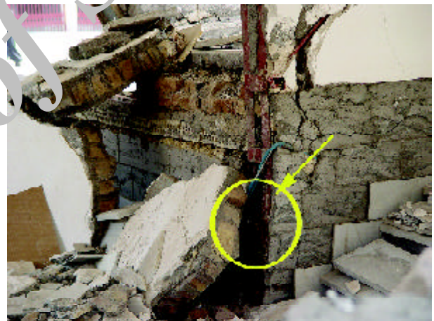
Figure17. Weld rupture in battens of batten column in an insurance building
