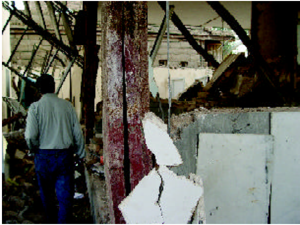
Figure 1. Rupture of longitudinal joint in box column.
