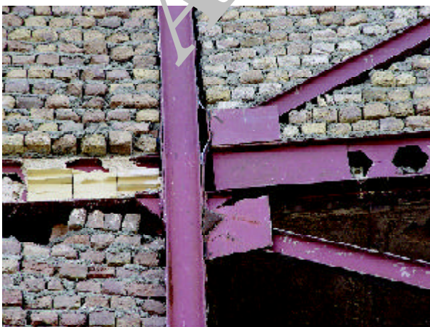
Figure 7. Separation of connection plate of batten column.
