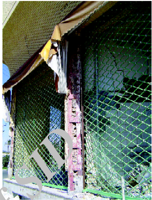
Figure 9. Overall buckling of batten columns about hollow axis in a store.
