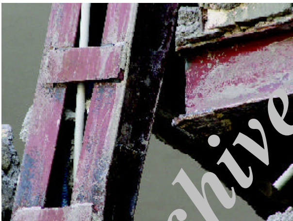
Figure 6. Rupture of seat angle of simple connection.
