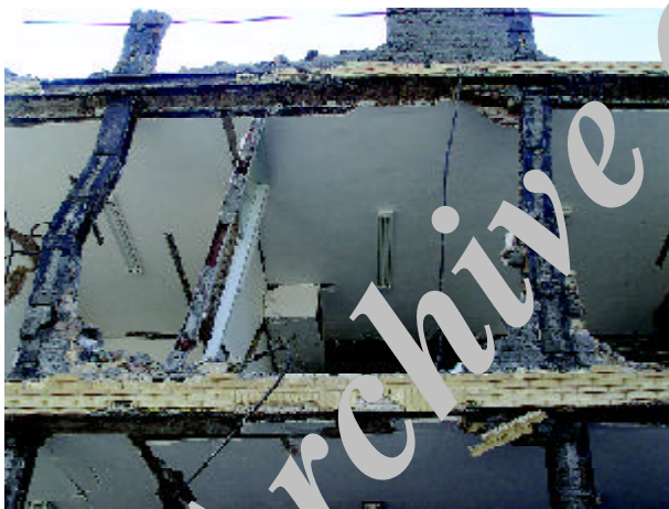
Figure 8. Overall buckling of batten columns about hollow axis in a pharmacy.
