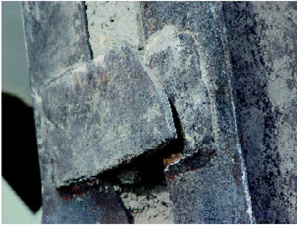
Figure13. Rupture of battens in a pharmacy.
