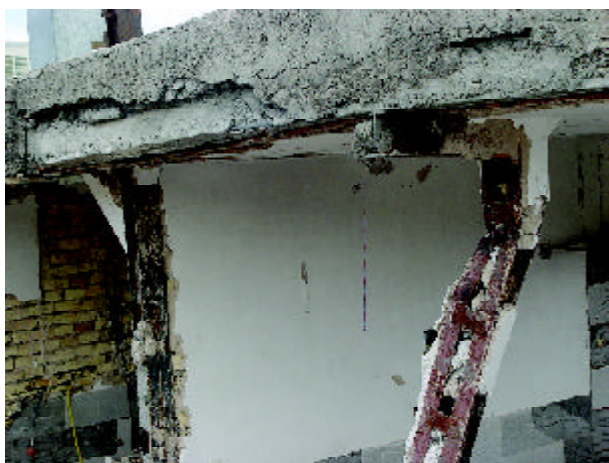
Figure 11. Lateral-torsional buckling of batten column in a store building.
