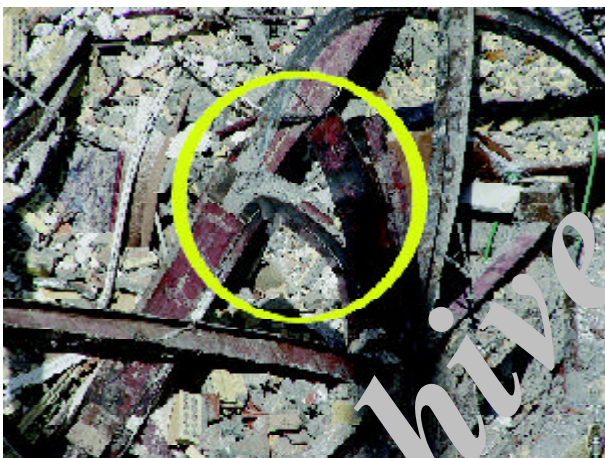
Figure19. Failure of batten column at splice location in kimia building.
