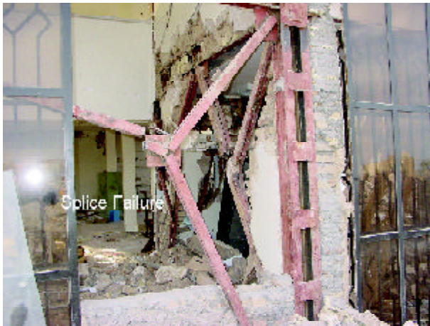
Figure 20. Fracture of spliced bracing members.
