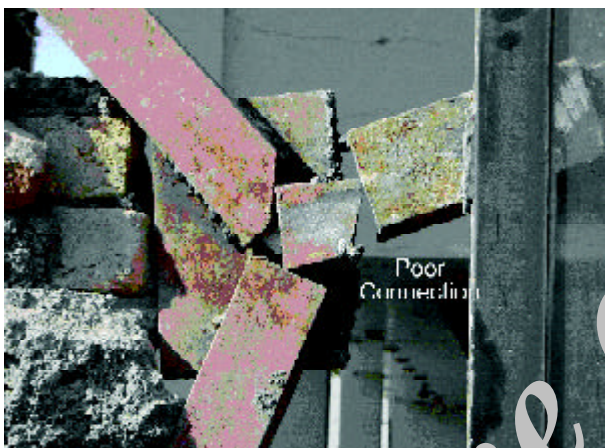
Figure 21. Very poor bracing connections.
