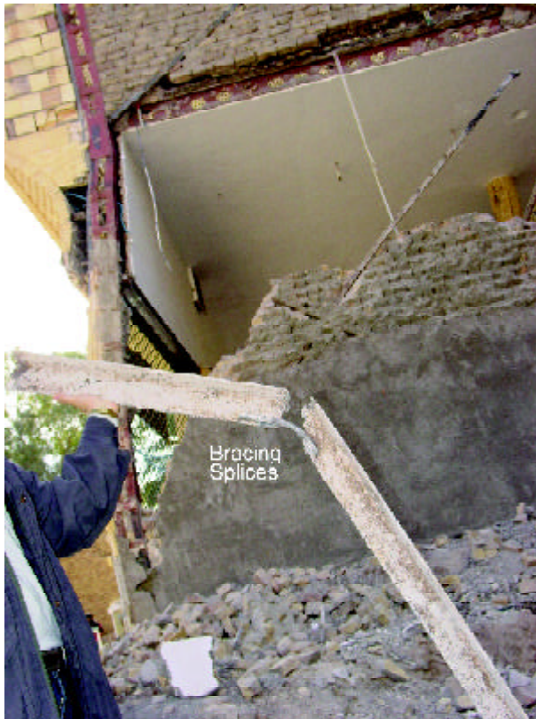
Figure 9. Brace spliced with a rod.
