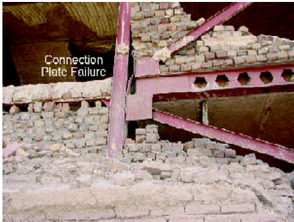
Figure 14. Fracture of bracing-to-frame connections.
