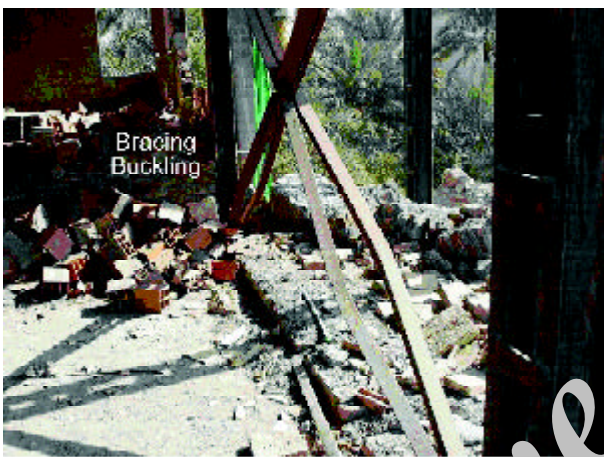
Figure 26. Out of plane buckling of built up brace.
