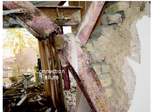
Figure 22. Fracture of bracing connections.
