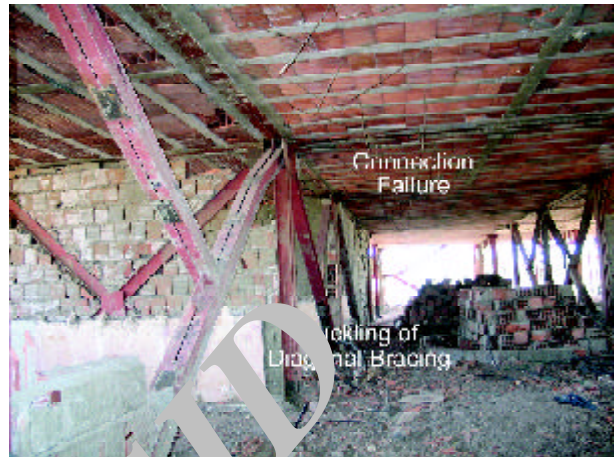
Figure 17. Buckling of diagonal bracings.
