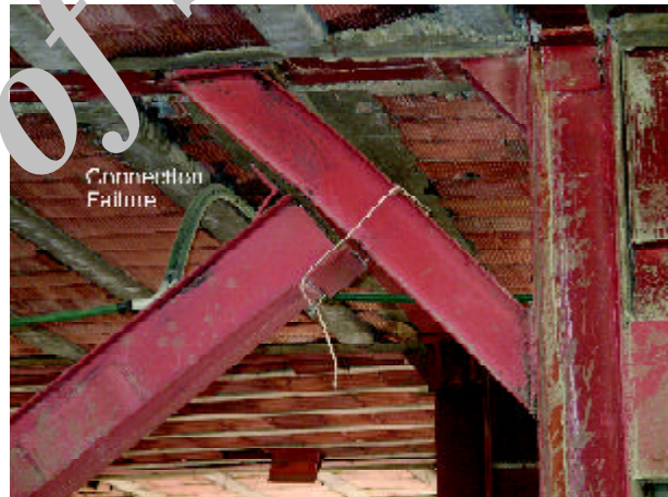
Figure 18. Failure of bracing connections to frame.
