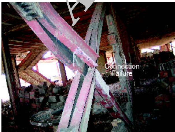
Figure 16. Failure of cross bracing connections.
