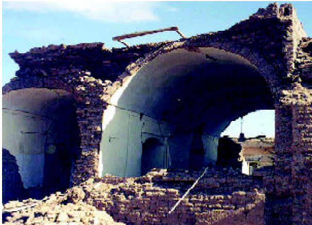
Figure 4. Survival of masonry vault roof during the earthquake.
