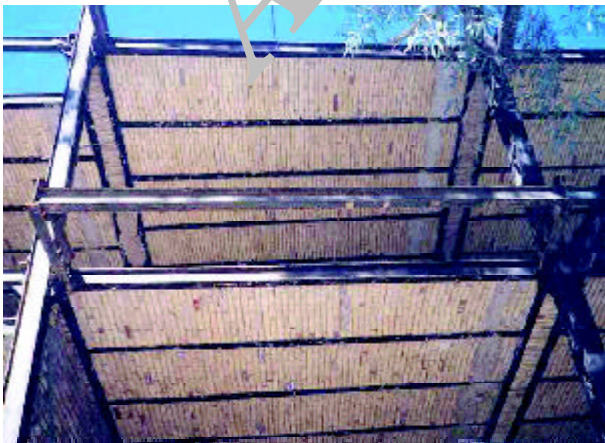
Figure 15. Good seismic performance of anchored jack arch slabs made with lightweight perforated bricks.
