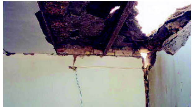
Figure 6. Collapse of masonry arches due to the movement of end support wall.
