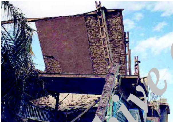
Figure 10. Integrity of the anchored jack arch slab under earthquake loading and after collapse.
