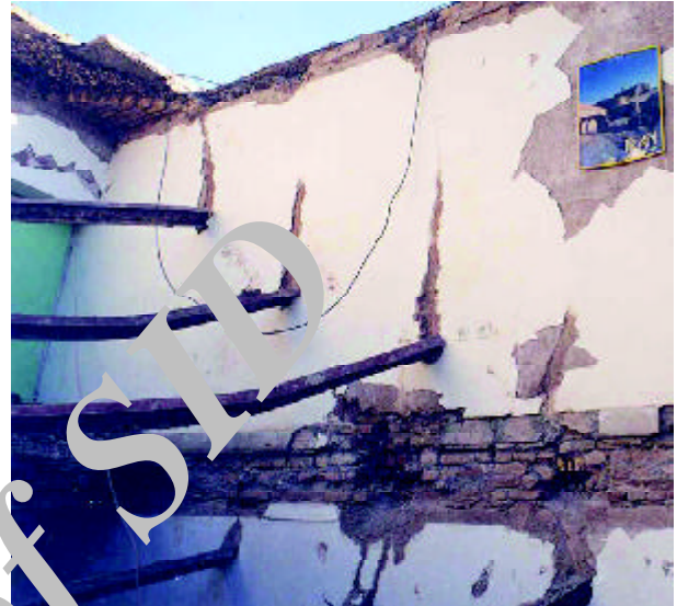
Figure 5. Collapse of jack arch steel beams as a result of small bearing length.
