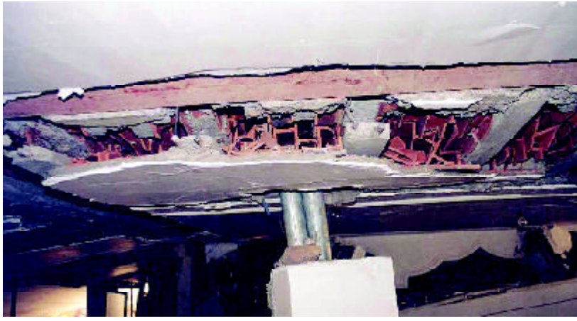
Figure 18. Lack of proper connection between the slab concrete beams and the steel support beam.
