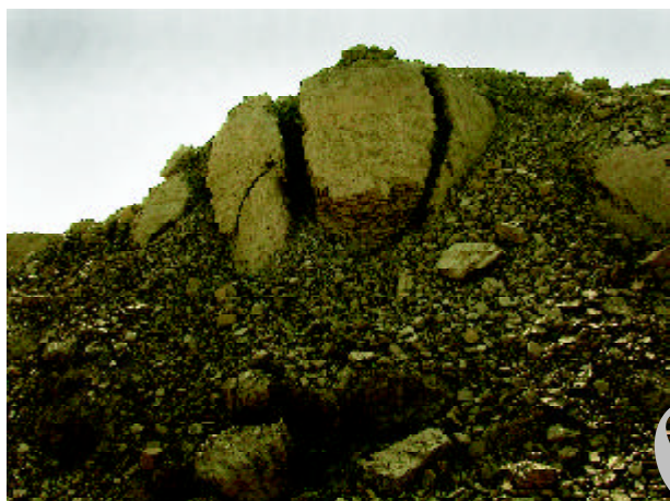
Figure 16. Collapsed round turret on the ramparts that shows evidence of having burst apart from collapse of internal layers.
