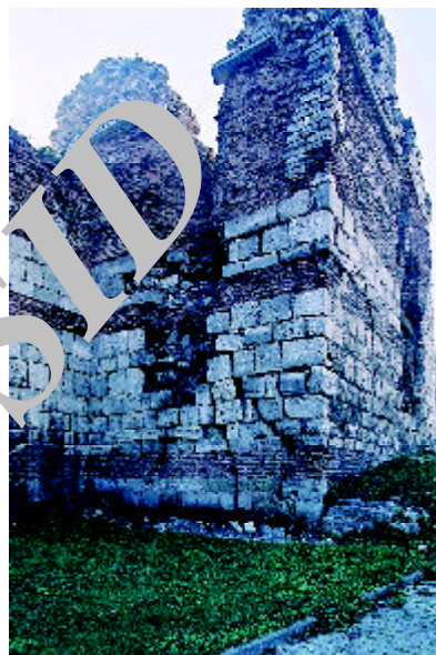
Figure 26. Surviving portion of the original Istanbul city walls. The cracks and broken section pre-dated the 1999 earthquake.
