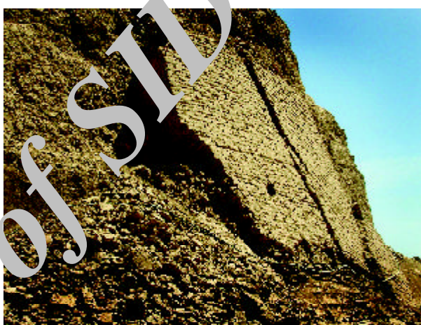
Figure 7. View of collapsed outer walls of a round tower. The Khesht construction of the outer layer has fallen off of the earlier inner layers that are most likely a combination of periods of building in different methods.
