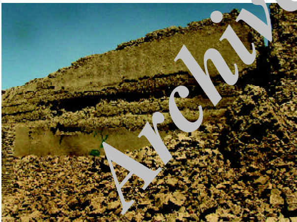
Figure 24. South-facing outside wall of the stables courtyard showing how the layering of the chineh walls has interrupted the cracking and collapse of sections of the wall, thus helping to maintain the stability of the partly undermined upper part of the wall.
