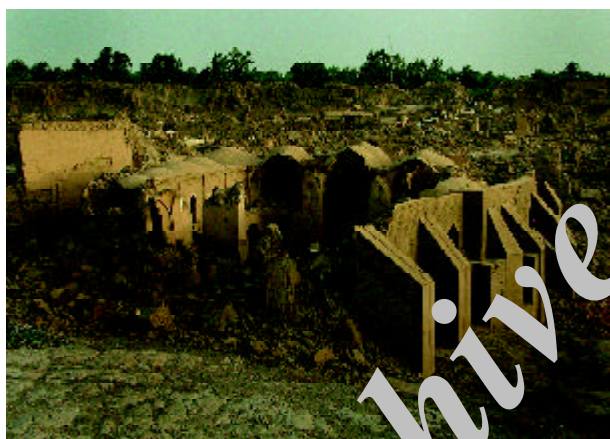
Figure 19. The ruins of the Caravansary show that the domed rooms on the second level behind the buttresses have collapsed, while the ones opposite still remain. There are no buttresses behind the external wall of the opposite side. The base of the 5th buttress is crushed.
