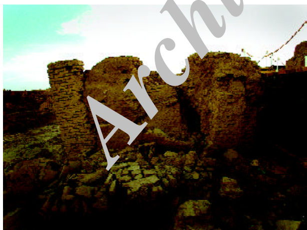
Figure 17. A massive pier composed of different periods and types of Khesht and chineh construction that have separated from each other during the earthquake.
