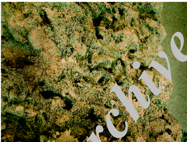
Figure 2. Evidence of termite damage in a wall of the Arg-e Bam showing extensive deposits of frass with insect tunnels.
