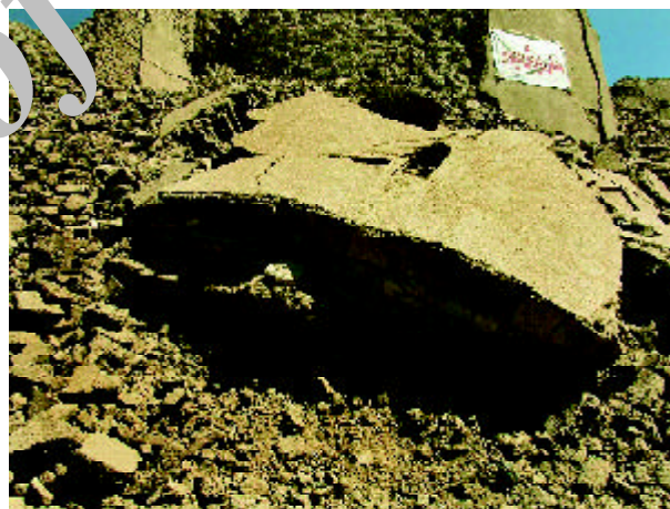
Figure 22. Collapsed section of the main gateway showing imbedded timber reinforcement of the Khesht wall.
