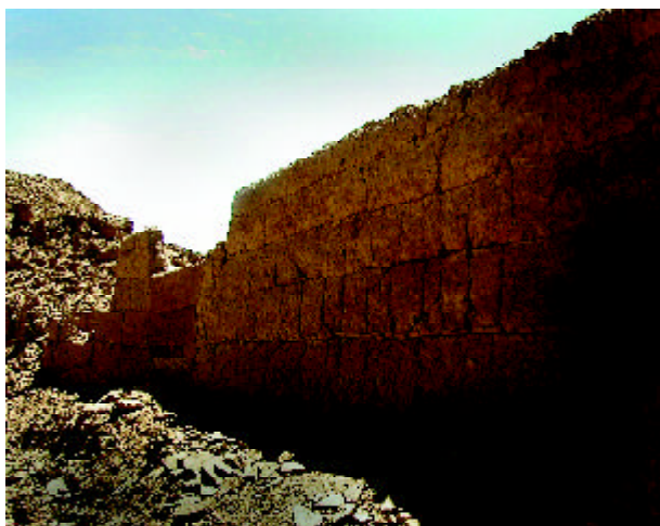
Figure 5. Chineh wall inside the Arg-e Bam that was only slightly damaged in the earthquake.
