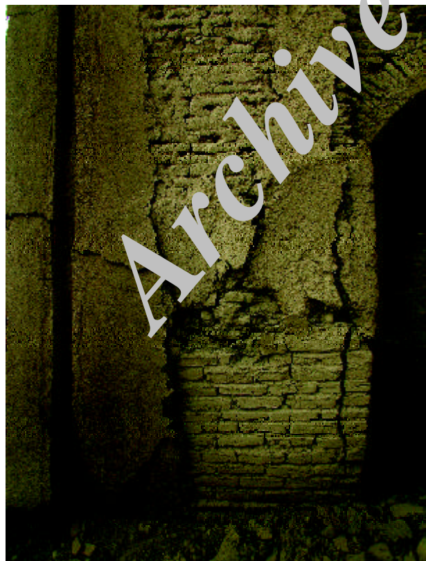
Figure 8. Pier in a partially collapsed section of the Caravansary showing the bursting of the outer layers from internal expansion from the earthquake vibrations.
