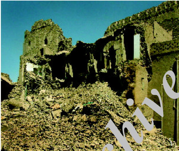
Figure 14. Buildings above the Stable Courtyard that collapsed from the lateral spreading failure of the retaining wall and fill beneath.
