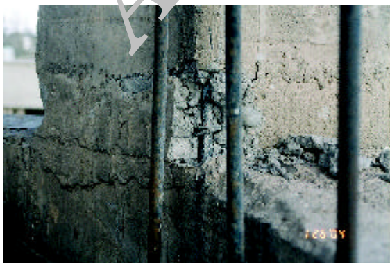
Figure 1. Elevated concrete water tank located in near the old section of the city where the damage was high. The tank experienced severe stress and deformation at the column-beam connections.
