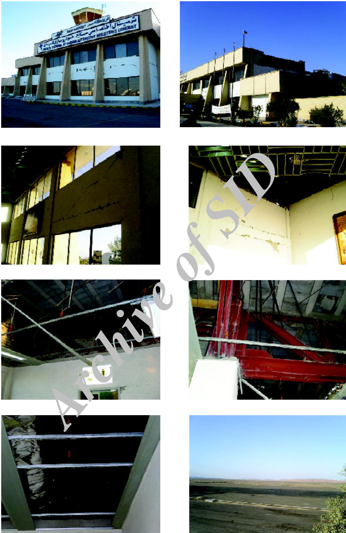
Figure 12. The engineered steel frame terminal building at Bam airport was moderately damaged. The masonry infill walls were damaged. The false ceilings were severely damaged. The airport runway had little damage.
