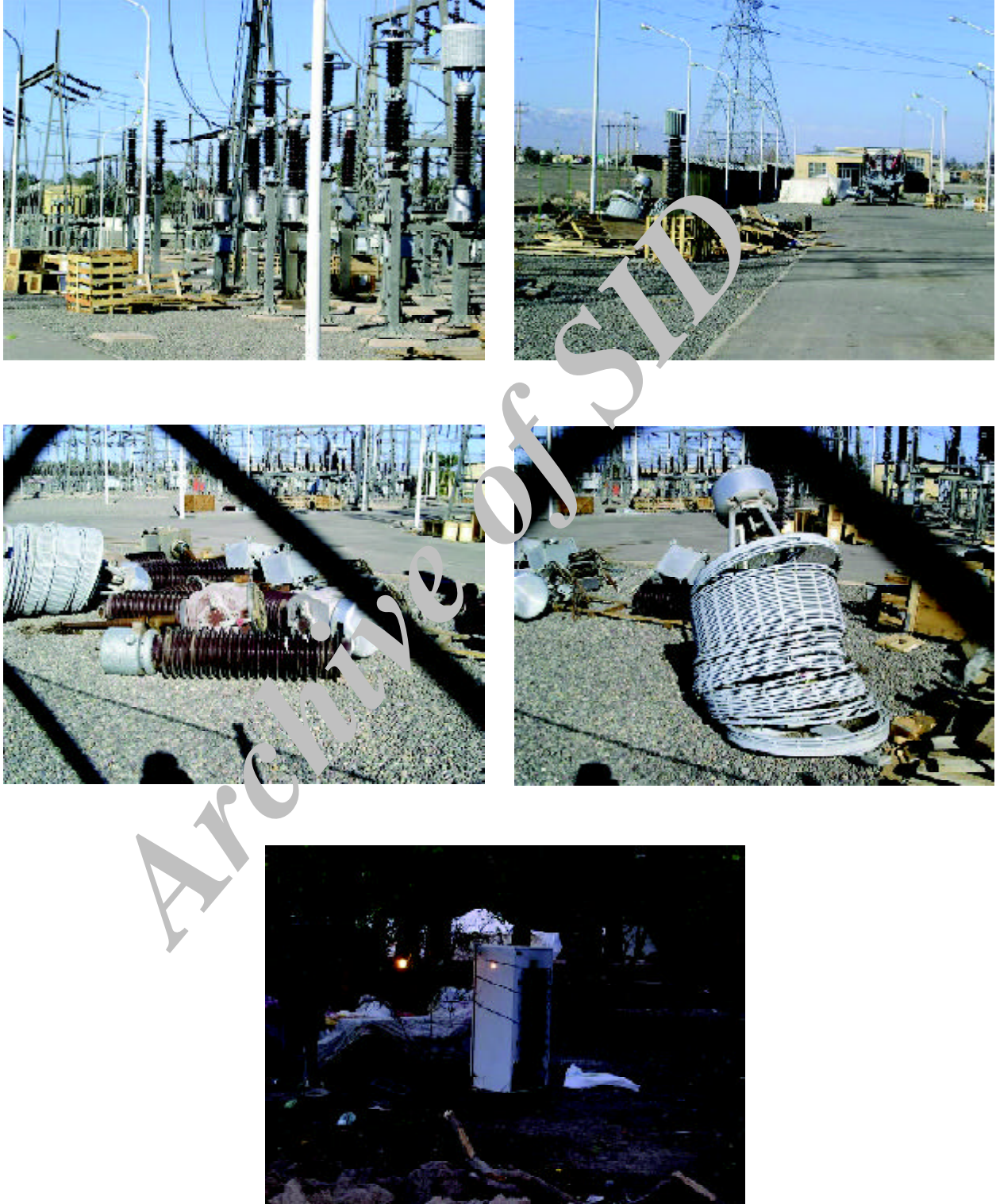
Figure 9. Damage to various electric equipments in the 230kV substation is observed in the above pictures. At the time of our visit (one month after earthquake) the electricity was available throughout the city, even though most of the users' buildings had been severely damaged to use the electricity.
