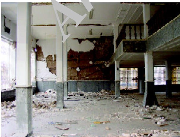
Figure 24. Severely damaged gypsum layer finishing of the interior wall of the Bank Refah Karegaran building (Photo by M. Hosseini).
