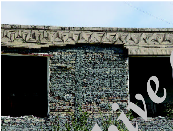
Figure 14. Failure of the brick facade on the external wall of a residential building - Note to the popped out windows as well (Photo by M. Hosseini).
