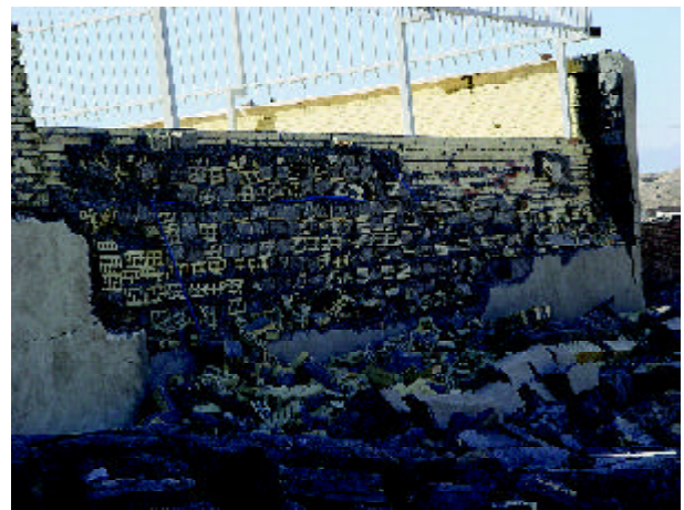
Figure 16. Damage to the plastered brick and block facade in a yard wall (Photo by M. Hosseini).
