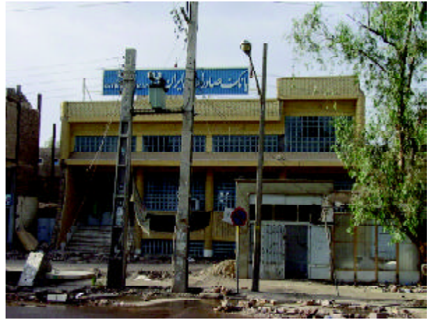
Figure 35. Damage to the glasses of widows in Bank Saderat Iran building (Iran Import Bank) (Photo by M. Hosseini).
