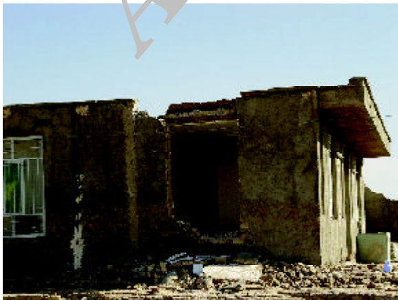
Figure 44. A popped out window in a one story residential building (Photo by M. Hosseini).
