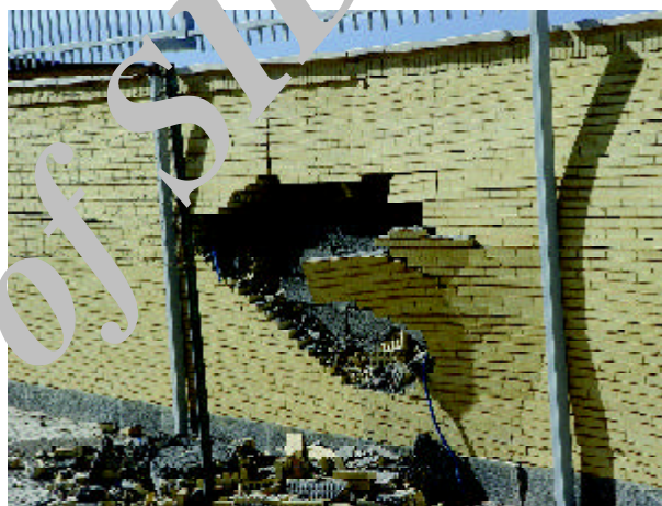
Figure 13. Damage to the brick facade in a yard wall (Photo by Mahmood Hosseini).
