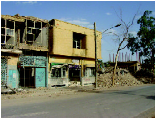
Figure 37. Damage to the glasses of widows in the second story of a residential building (Photo by M. Hosseini).
