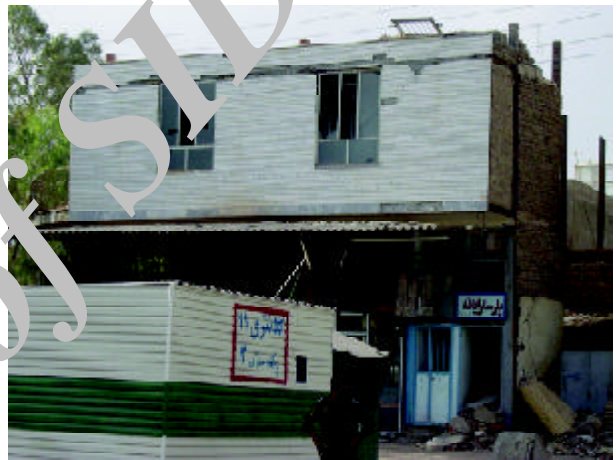
Figure 36. Damage to the glasses of widows in the second story of a residential building - Note to that horizontal damage line in the façade at the level of roof (Photo by M. Hosseini).
