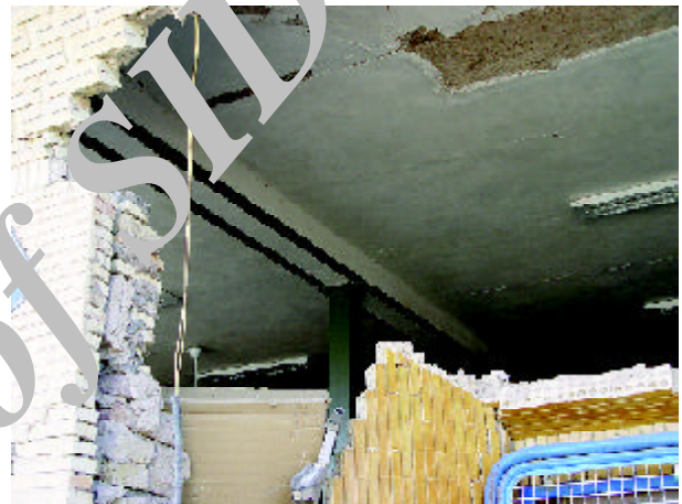
Figure 9. Severely damaged interior partition (Photo by M. Hosseini).
