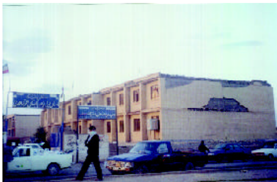
Figure 10. Damage to the so called 3cm brick facade in the second story of the Hijab girls' mid school (Photo by M. Hosseini)
