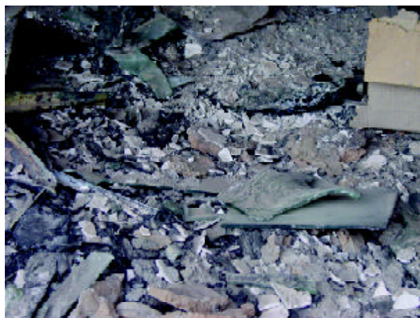
Figure 50. The deformed pieces of glass due to the fire occurred in the shop shown in Figure (49) (Photo by M. Hosseini)
