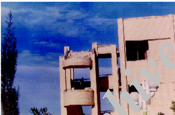
Figure 19. Damage to the staircase roof in the three story building of Azadi Hotel (Photo by M. Hosseini).
