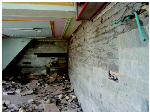
Figure 27. Severely damaged stone tile finishing of the interior wall of the Bank Refah Karegaran building (Photo by M. Hosseini).
