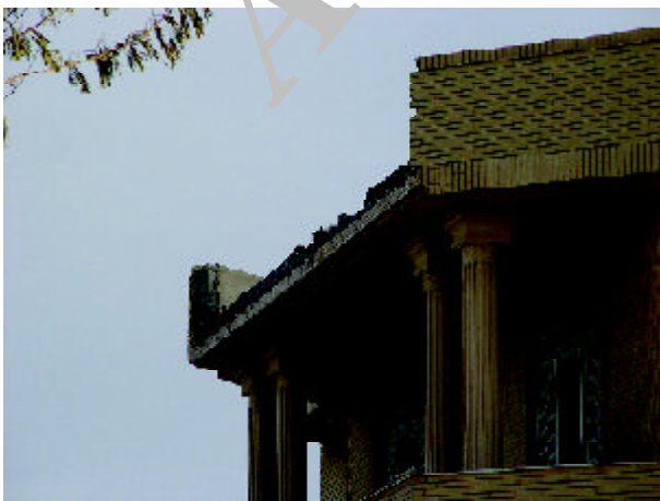
Figure 39. Partial collapse of parapets in a two story building (Photo by M. Hosseini).
