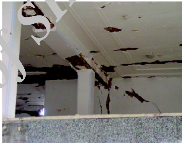
Figure 26. Severely damaged gypsum layer finishing of the ceiling of the Bank Refah Karegaran building (Photo by M. Hosseini).
