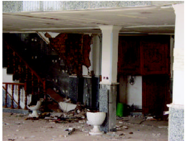
Figure 25. Severely damaged gypsum layer finishing of the interior wall of the Bank Refah Karegaran building (Photo by M. Hosseini).
