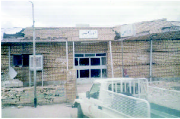
Figure 32. Damage to the glasses of widows in the Emergency Section of the city hospital (Photo by M. Hosseini).
