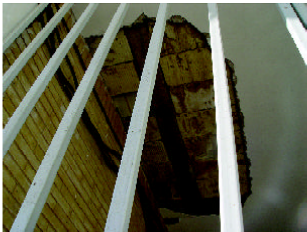
Figure 28. A big part of gypsum veneer of the ceiling has separated and fallen (Photo by M. Hosseini).
