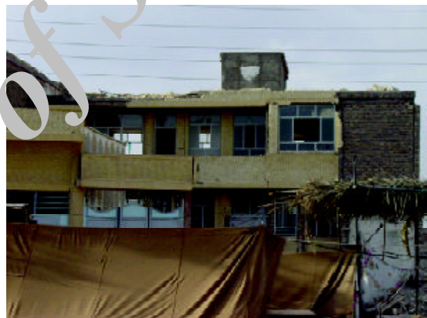
Figure 40. Complete collapse of parapets in a two story building (Photo by M. Hosseini).
