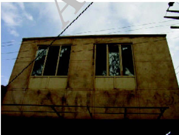
Figure 34. Damage to the glasses of widows in the second story of a residential building (Photo by M. Hosseini).
