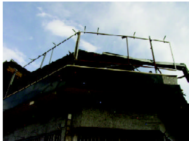
Figure 41. Collapse of tablets and bill boards in a commercial building (Photo by M. Hosseini).
