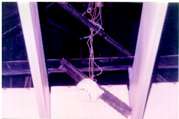
Figure 46. The failed smoke detector of the Bam airport (Photo by M. Hosseini).
