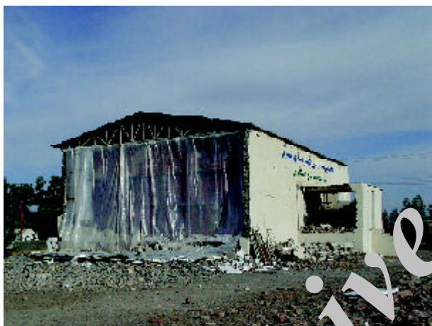
Figure 2. Complete collapse of the external wall of the refrigeration saloon of Khormayyeh Shargh (east date) export company made of concrete block masonry (Photo by M. Hosseini).
