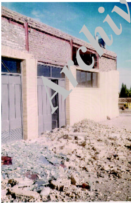
Figure 12. Damage to the brick facade in the top part of the walls in the logistic building of Azadi Hotel (Photo by M. Hosseini).
