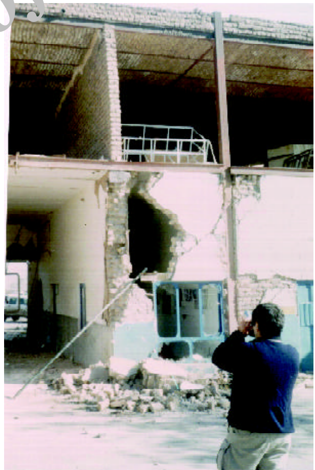
Figure 1. Collapse of the external walls made of brick masonry in Emdad Khodro building (Photo by M. Hosseini).
