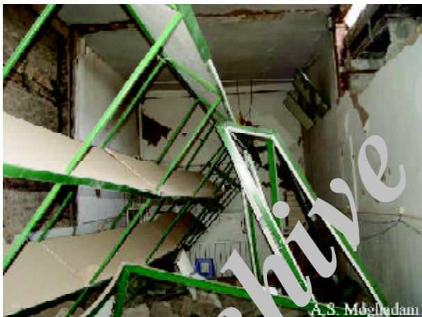
Figure 52. The toppled shelves of a shop board due to their weak connection (Photo by A.S. Moghadam).
