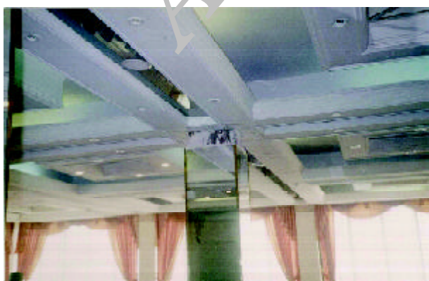
Figure 29. A sample of damages to the veneers of the columns tops in Azadi (Iran Parsian) hotel (Photo by M. Hosseini)
