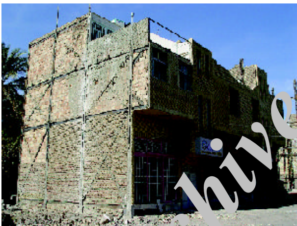
Figure 38. Collapse of parapets in the Iran Insurance Company building (Photo by M. Hosseini).
