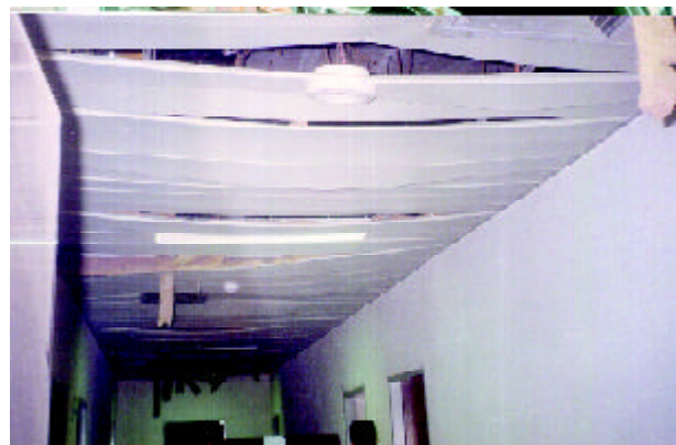
Figure 22. The deformed parts of the false ceiling in the Bam Airport Terminal Building (Photo by Mahmood Hosseini).
