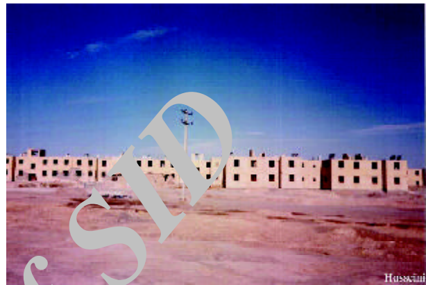
Figure 21. Severely damaged or totally collapse penthouses in the residential complex two story buildings (Photo by M. Hosseini).
