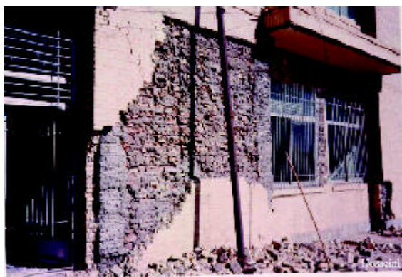
Figure 11. Damage to the so called 3-cm brick facade in the first story of the office building of the city electric substation (Photo by M. Hosseini).
