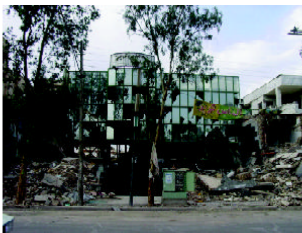
Figure 31. Damage to the glass facade of trade and tourism building (Photo by M. Hosseini).
