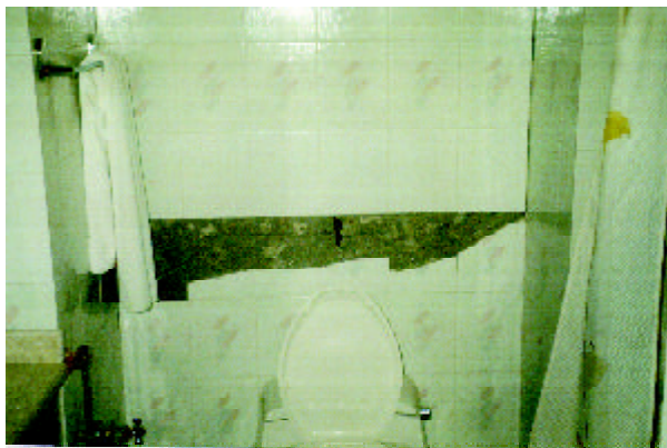
Figure 30. A sample damages to the ceramic tile interior veneers in the bath rooms of Azadi (Iran Parsian) hotel (Photo by M. Hosseini).
