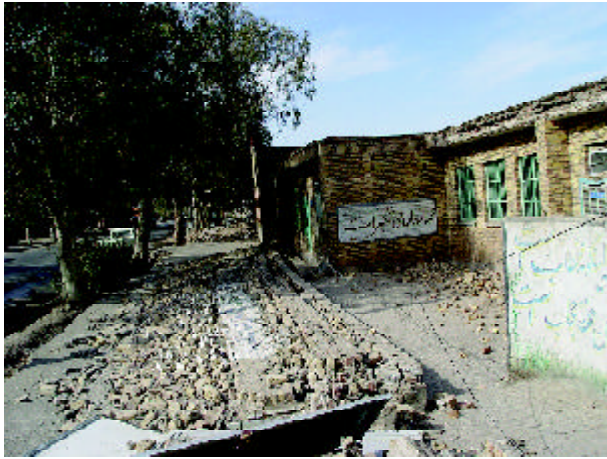
Figure 6. Topped brick wall - Note to the fallen parapets as well (Photo by M. Hosseini).
