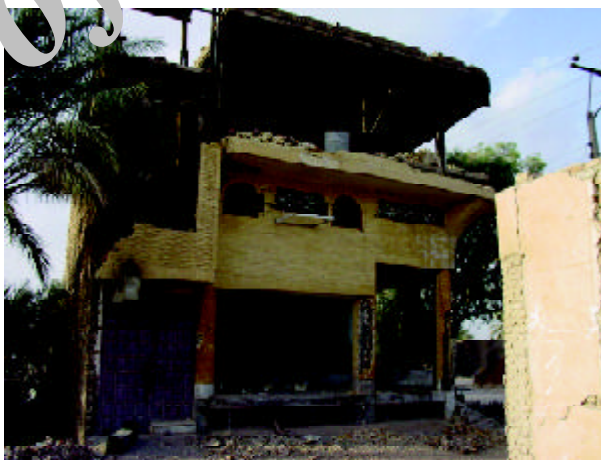
Figure 5. Collapse of the external wall masonry in the second and third stories of a 3 story steel structure building - the roof parapet has fallen as well (Photo by M. Hosseini).
