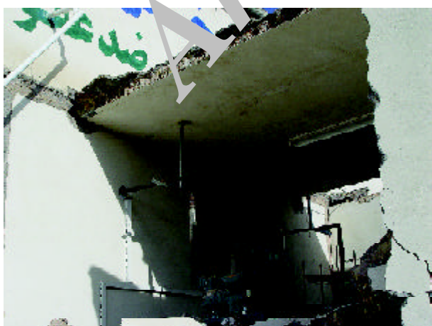
Figure 3. Complete failure of the external wall with partial collapse of the ceiling in the motor house of Khormayyeh Shargh export company (Photo by M. Hosseini).
