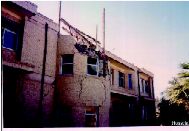
Figure 18. Severely damaged staircase roof in the office building of the city electric substation-Note to the broken glasses as well (Photo by M. Hosseini).
