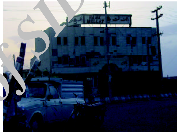
Figure 17. Damage to the stone tiles facade in Bamk Mellat building (Photo by M. Hosseini).
