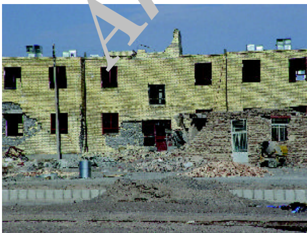
Figure 15. Damage to the brick facade in lower part of the two story residential buildings - Note to the collapsed penthouse as well (Photo by M. Hosseini).
