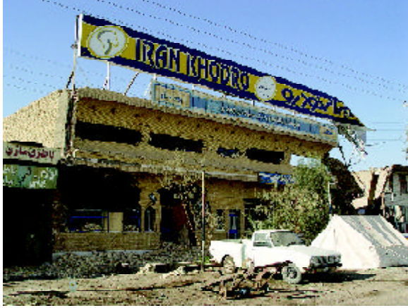
Figure 42. The windows in Iran Khodro building popped out of walls (Photo by Mahmood Hosseini).
