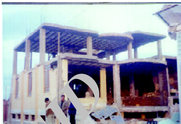
Figure 4. Collapse of external walls in an under construction R/C building, whose skeleton remained intact after the quake - Note to the fallen out window as well (Photo by M. Hosseini).
