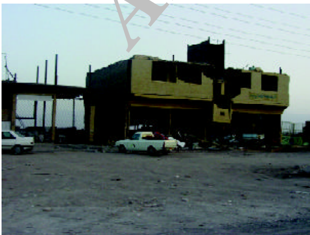
Figure 20. Severely damaged staircase in a commercial building (Photo by M. Hosseini).
