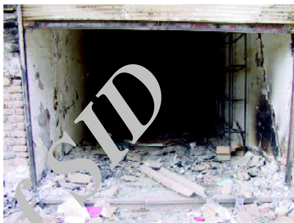
Figure 49. A partially burnt shop which got in fire because the failure of its electrical facilities (Photo by M. Hosseini).
