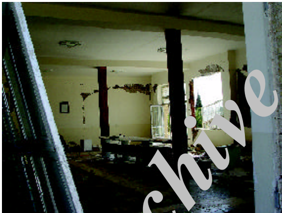
Figure 43. A popped out window in the electric substation office building (Photo by M. Hosseini).
