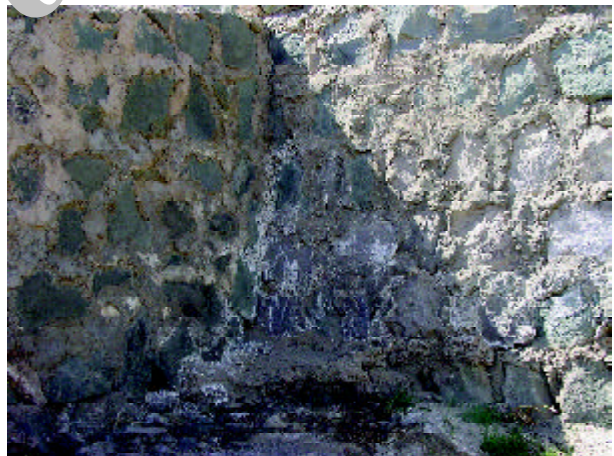
Figure 8. Leakage of water from tank wall.
