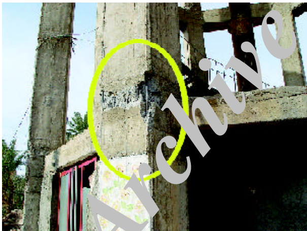
Figure 4. Inaccurately detailed cracked RC column [1].
