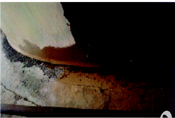
Figure 20. Damage to tank foundation due to tank uplift.
