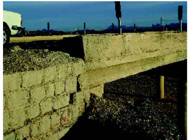
Figure 12. Settlement of Darzin bridge abutment.
