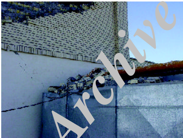
Figure 25. Damage to air conditioners.
