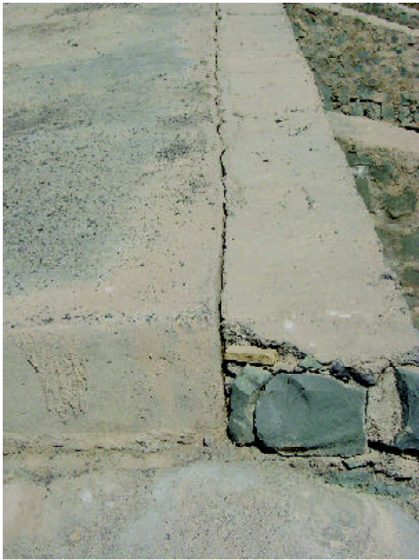
Figure 9. Cracks observed at construction joints of surrounding wall
