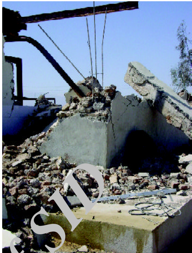
Figure 7. Collapse of chlorination building.
