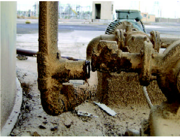
Figure 19. Rupture of pipe connections.
