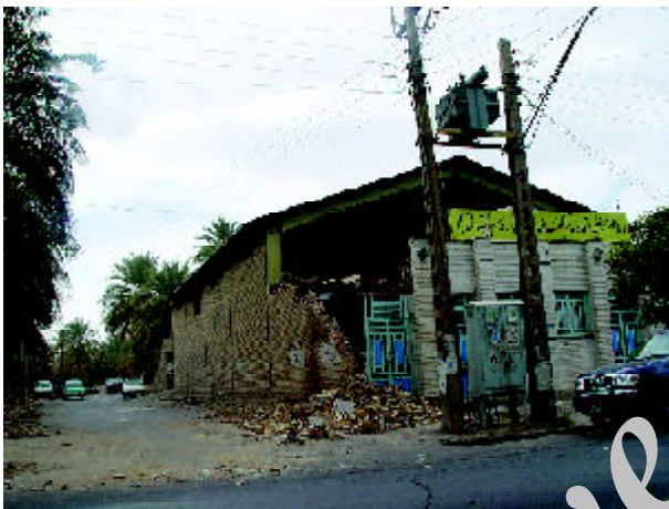
Figure 13. Damage to annex building of an industrial plant [1].
