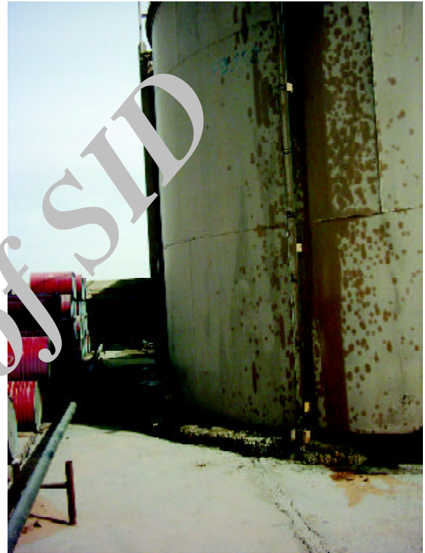
Figure 18. Leakage of oil from tank due to sloshing [1].
