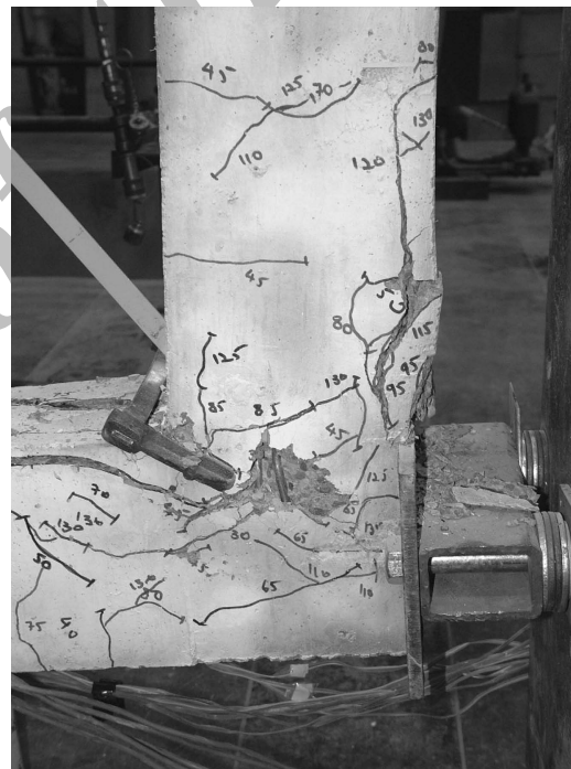
Figure 6. Pattern of cracking in the moment frame F1.
