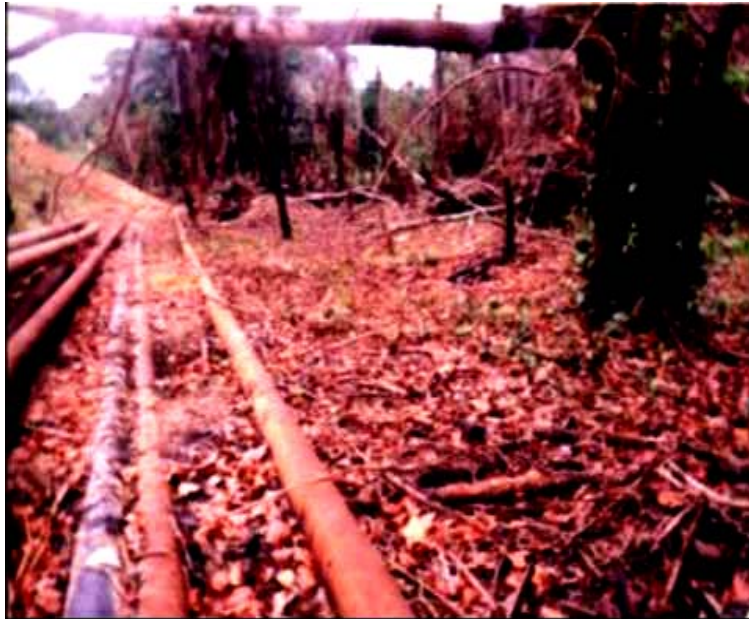
Fig. 2: A section of the study site showing pipelines, mangrove litters and felled tree forms within the right of way
