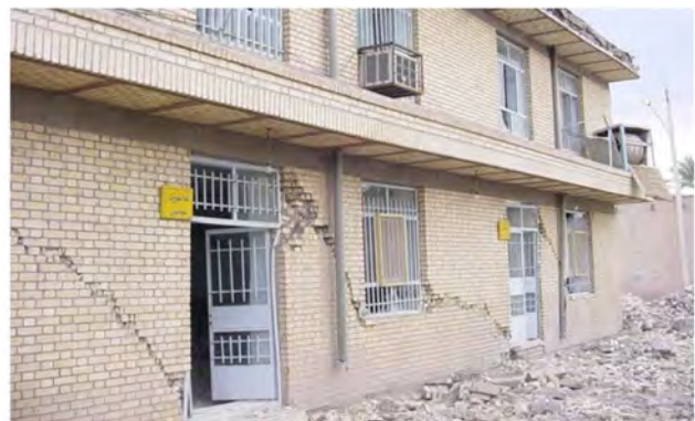
Figure 3. A two-story CM building after the 2003 Bam earthquake in Iran.
