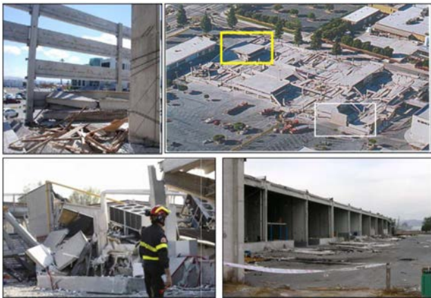
Figure 8. Precast concrete failures in past earthquakes.
