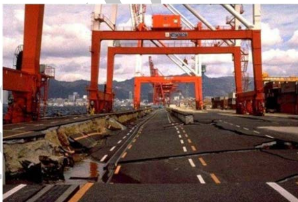
Figure 8. Lateral spreading damage to a quay wall (Kobe earthquake, 1995) [104].
