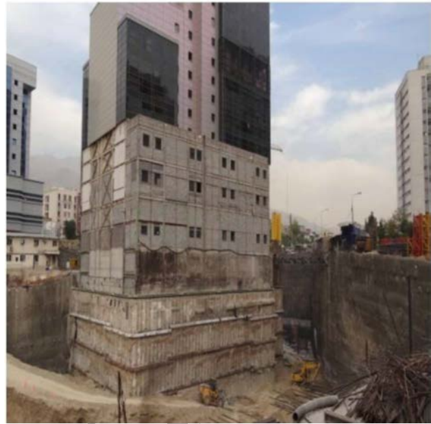
Figure 6. South and west views of the excavation, the retaining system and the existing tower; in this image, all 4 levels of wailing have been installed. Also the nailing system in other parts of the excavation can be observed.
