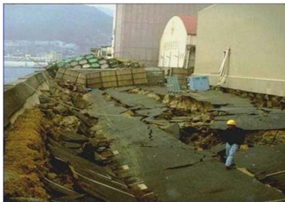
Figure 7. Lateral spreading damage to a quay wall (Kobe earthquake, 1995) [103].
