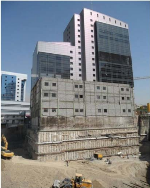
Figure 4. South and west views of the excavation including a view from the existing building.
