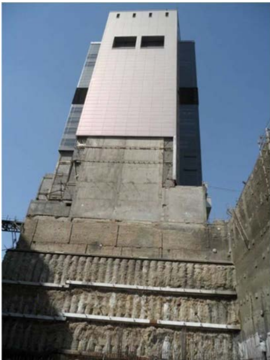
Figure 5. East view of the excavation including a view from the existing building.
