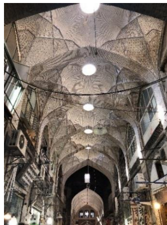
Fig 9. View of ceiling orifices
