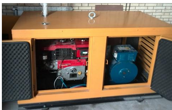
Figure 2- A general view of diesel generator
