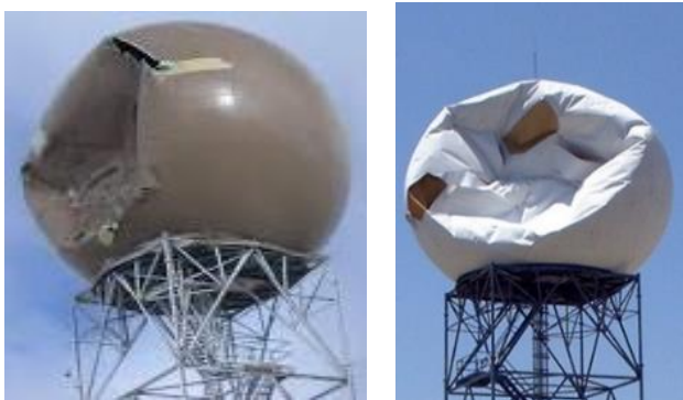
Fig. 12 Some damaged weather radome samples due to severe storms [15, 16]
