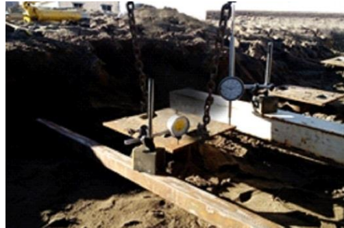
Fig. 1. The distance of installed piles in soil and application of displacement dial gauges
