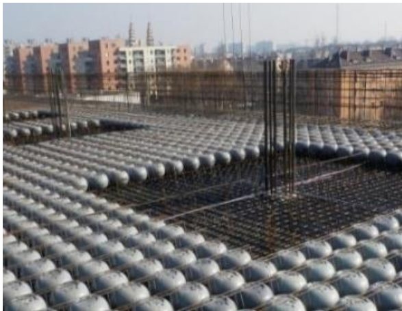
Fig. 1. A view of the implementation of the ceiling of the bubble slab
