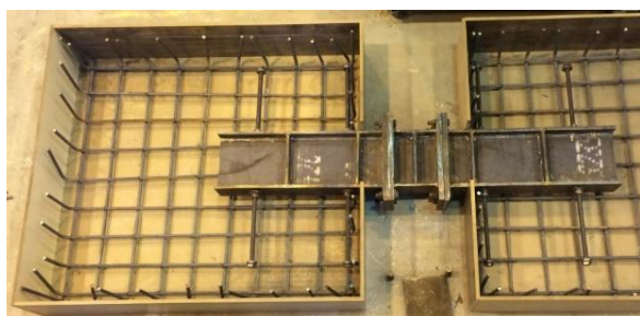
Fig. 4. Coupling Beam Embedded into RC Shear Wall (All Front Steel Reinforcements are not shown)
