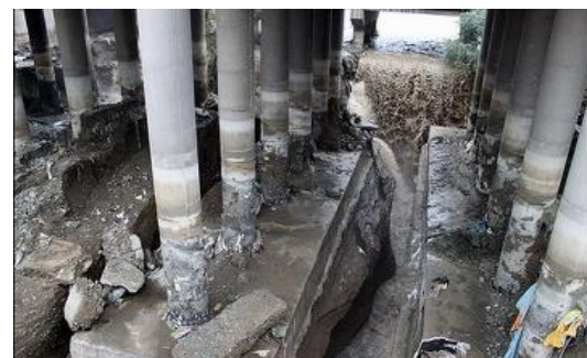
Fig. 2. Bridge Failures due to Scour (Kan Bridge)
