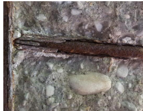
Fig. 1 Uniform corrosion in reinforcement (Bandar-e Mahshahr.)
