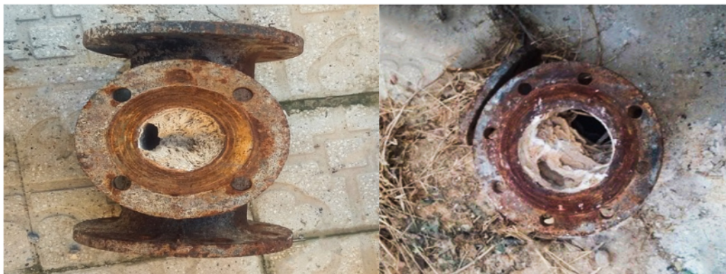
Fig. 9. Sedimentation formed on water distribution network components
