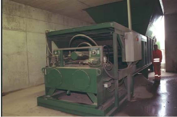
Figure 3-4.3: Hydraulic Unit of Waste Compaction Unit
