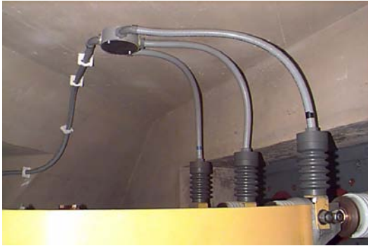
Figure 6. PD sensors - A2, B2, C2 on generator phase bus
