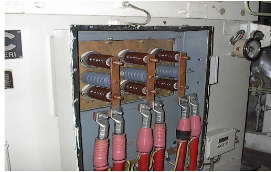
Figure 8 – 120 mm PD sensors inside motor box
