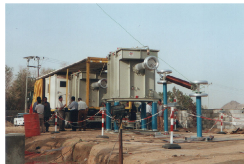
Fig. 10: Series connection of two reactors (Courtesy of CEPCO / Saudia Arabia)
