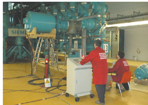
Fig. 7: "Shielded" ACRF circuit with SF 6 -insulated reactor during testing a 400 kV GIS (Courtesy of Siemens)
