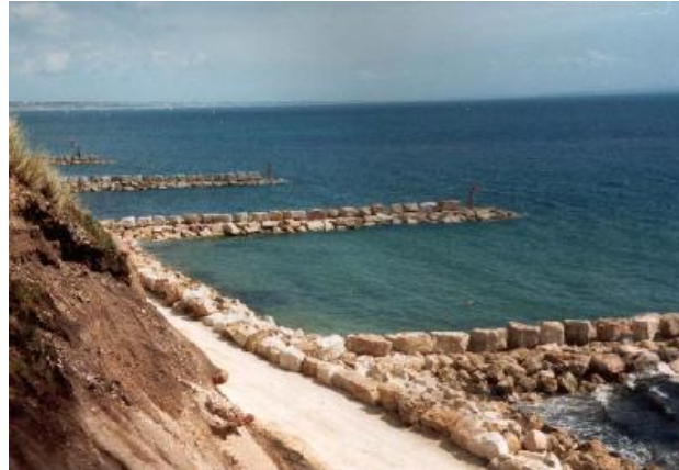
Fig1. Rock groins with temporary additional crest layer in place (Crossman et al, 2003).
