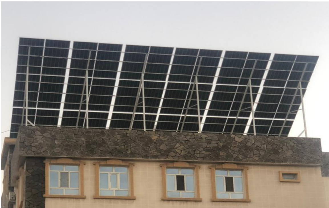
Figure 1- Solar panel on top of the roof of a residential building in the south part of the community mosque in Herat city. Source of research findings
