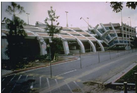
Figure 1: moment resistant frame failure
