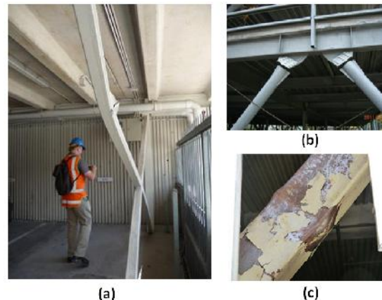
Figure 1: CBF failure from top down and left to right: (a) Buckled brace (Christchurch Earthquake); (b) Out-of-plane deformation and fracture of gusset plates (Tohoku Earthquake); (c) Local buckling in square-HSS brace (Tohoku Earthquake). [1, 2]
