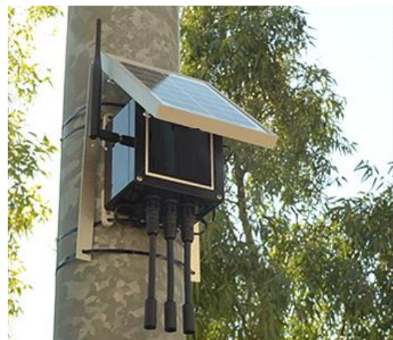
Figure 4 – Sensor box including temperature, humidity and carbon dioxide sensors, solar cell and telecom link
