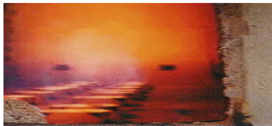
Furnace performance of ultra-burners after final modifications formed. Note the clean, compact flames
