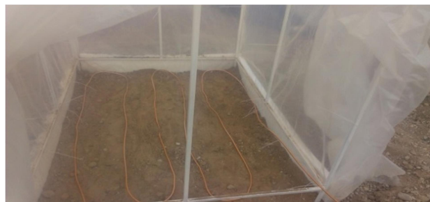
Fig. 3 Heat exchanger in greenhouse bed
