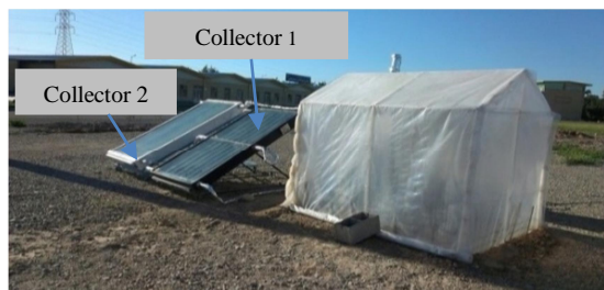
Fig. 2 Real view of greenhouse and heating system
